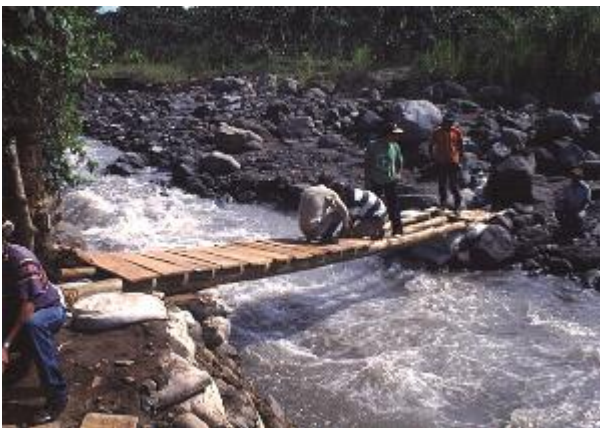
Figure 11 Rapidly constructed temporary foot bridge over the Rio Tambor, Finca Filadelfia. November 1998. Photo courtesy of William Rose.
