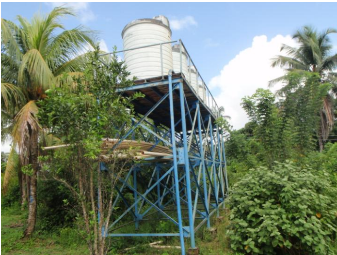
Figure 11. The water tower in Kayapaati and its polyethylene storage tanks.
