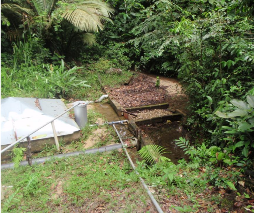
Figure 7. The intake for the water system at the time of evaluation, May 2010. The weir can be seen along with the gravel bed covering the intake in the center of the photo. The pyramidal structure in the left of the photo is the original slow sand filter.
